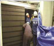
▼ 板式冷却器清洗/Plate Cooler Cleaning
