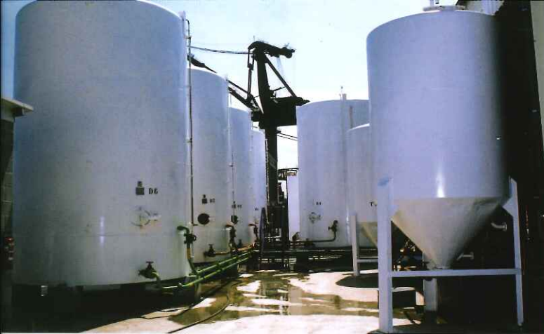
SLOP DISPOSAL PLANT
